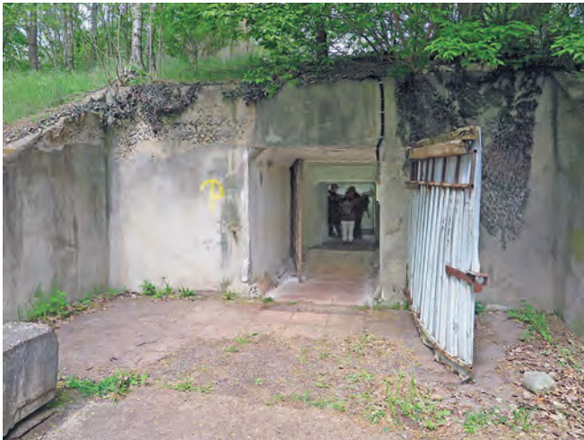
A rudimentary door now provides entry to the air defence HQ bunker Wünsdorf; in operational times this portal lay within a surface building. Photo Clive Penfold
